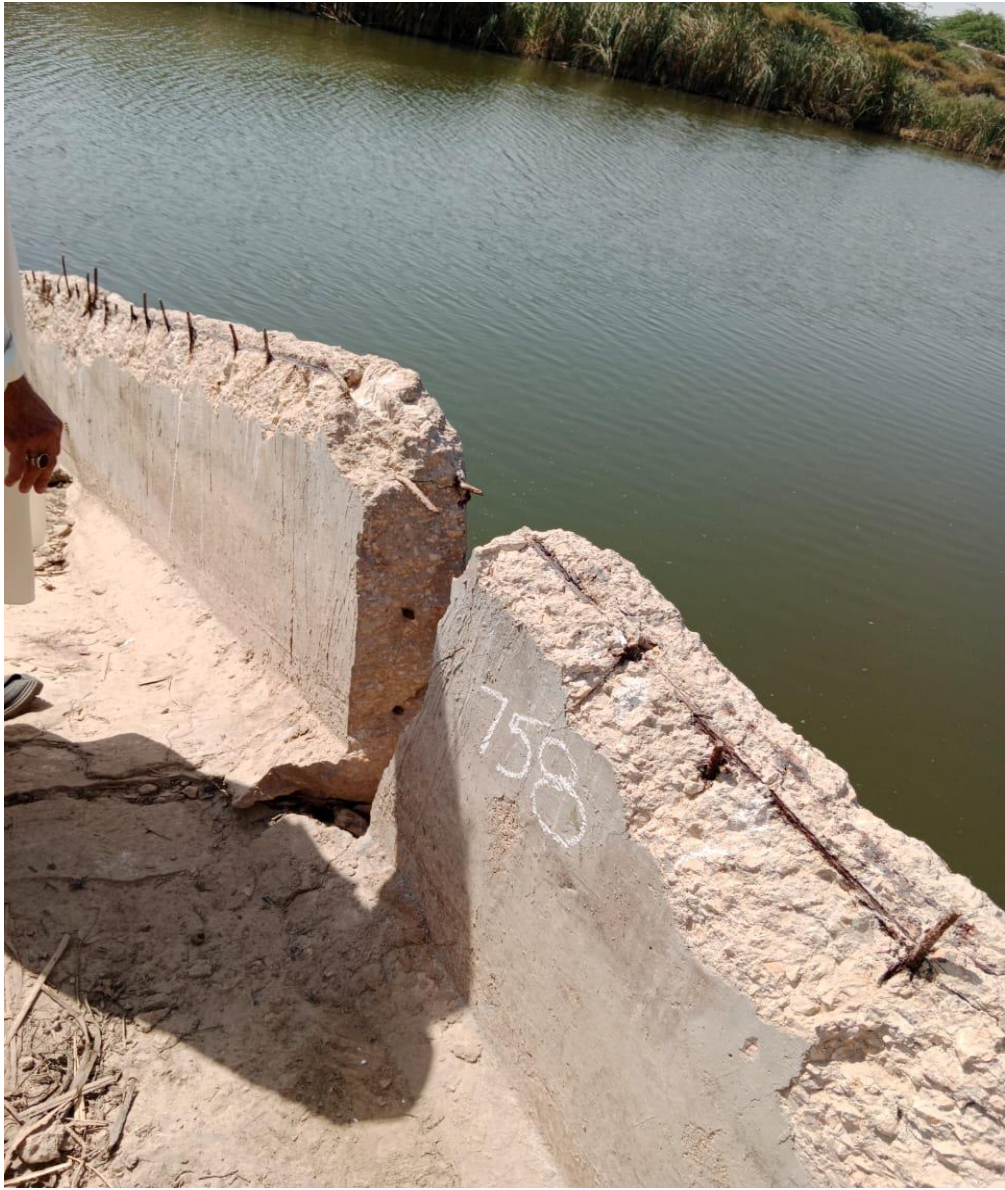
Collapse of Foot bridge at RD 758
